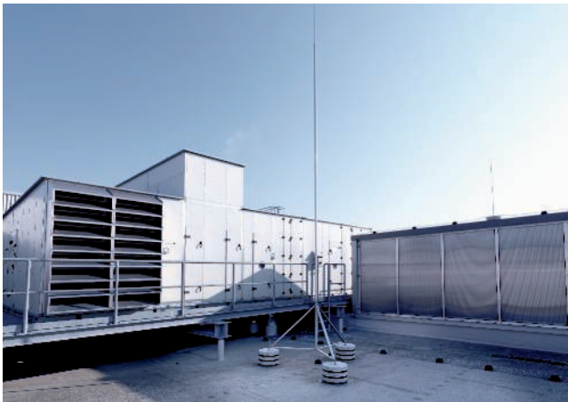
Insulated lightning protection with isFang
