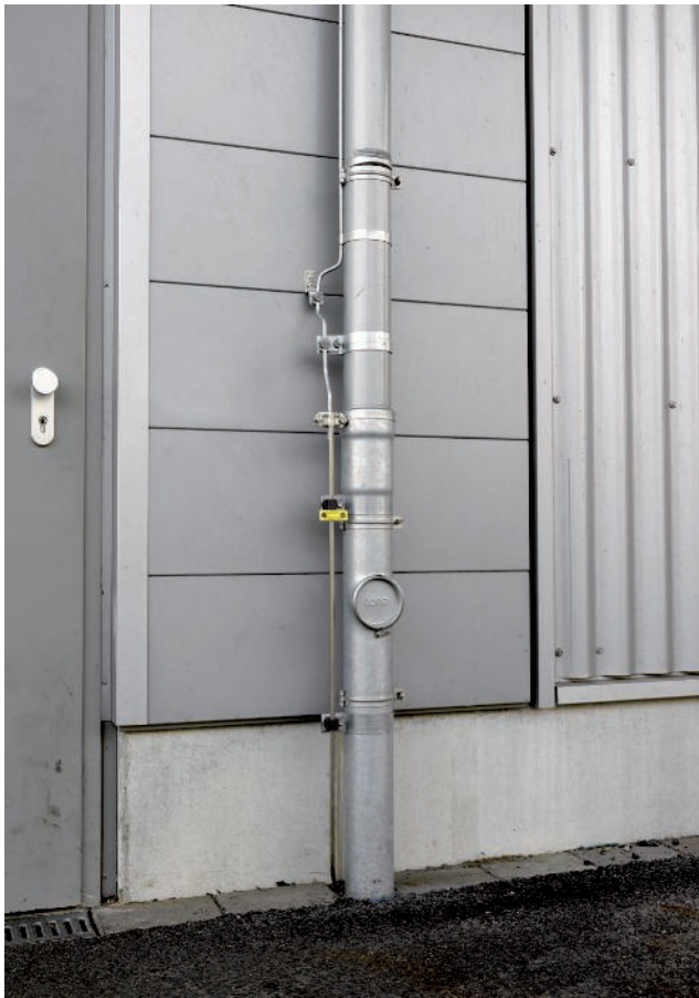
Lightning down-conductor at a downpipe
