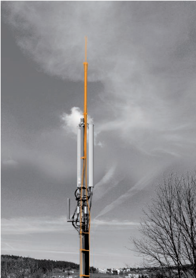
Cell tower with isCon® conductor
