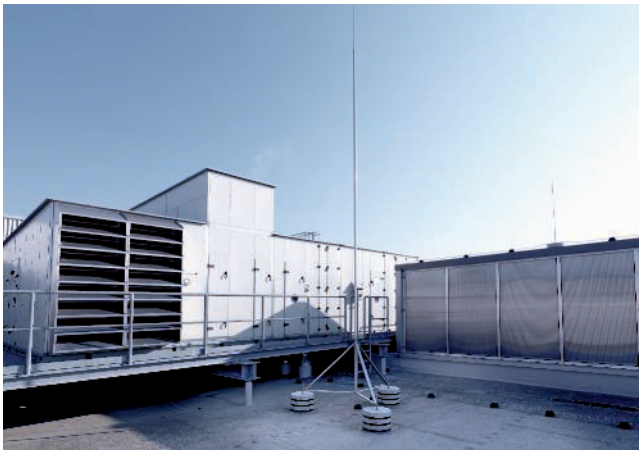
Aluminium air-termination mast
