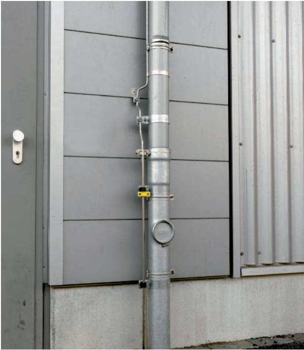
Lightning protection conductor on a rainwater downpipe
