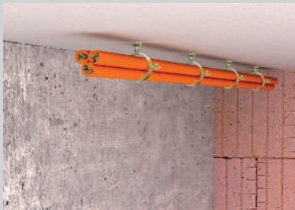
Bundled cable routing under the ceiling.
